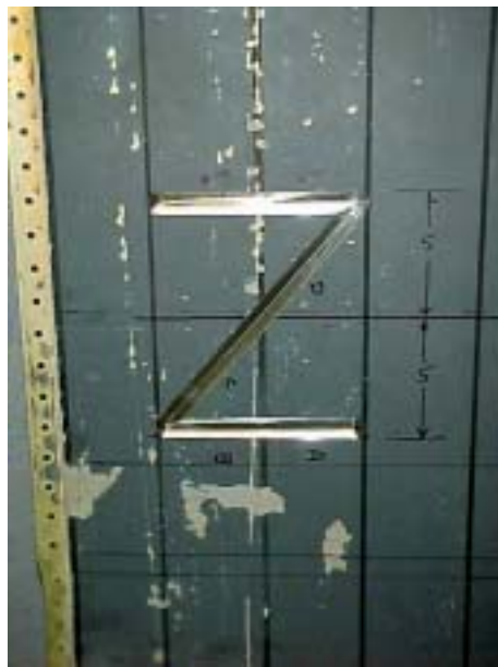
Figure 2. Centrally-located Milled “Z” damage.
